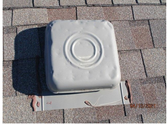
Roofing: Hail dents
