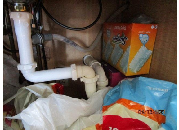
Plumbing: Drain assembly under kitchen sink
