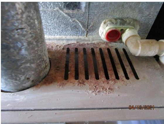
Heating: Corrosion/sediment on top of heater
