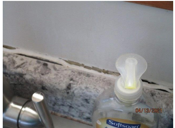
Kitchen: Recaulking needed along back of sink countertop
