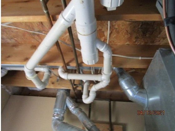
Plumbing: Plumbing and heat venting from hot water heater in utility room
